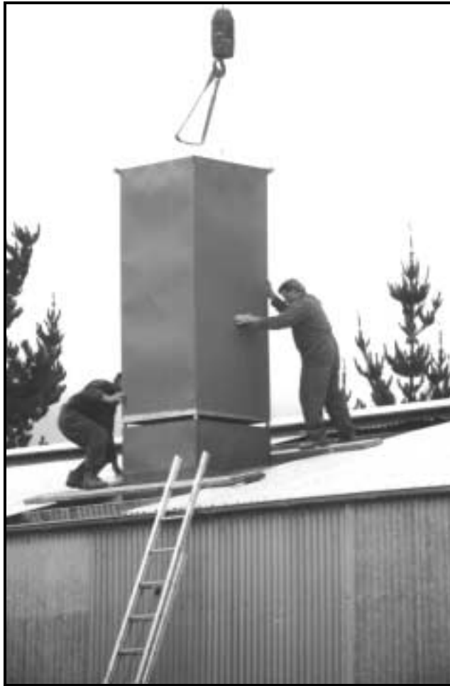
Photo 4-2 Exterior view of hood
